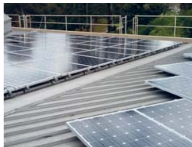
Figure 10 Part of photovoltaic system on the roof of the National Herbarium
